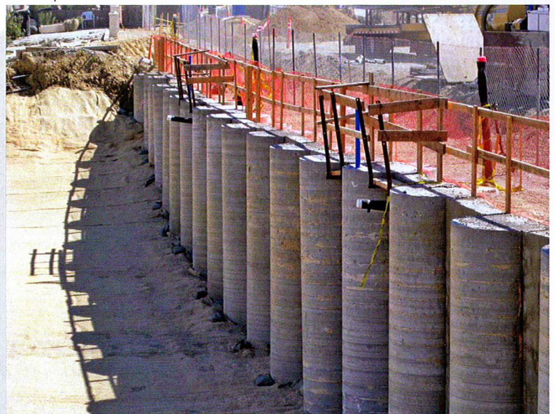
Phase 2 shear pin panel wall.
