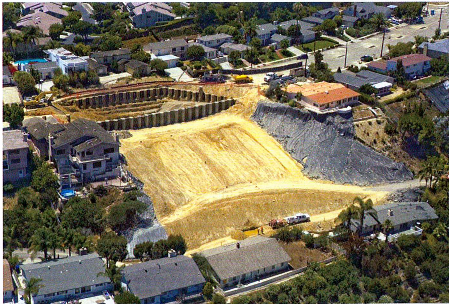
Phase 1 & 2 shear pin walls complete remedial slope grading and preparation for Phase 3.
